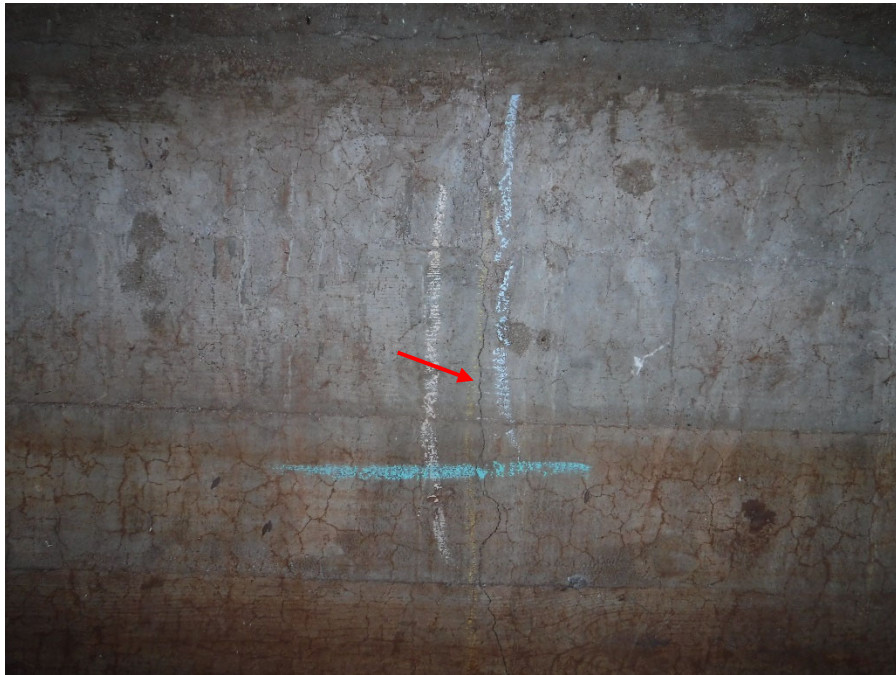
PHOTO 20 TYPICAL MODERATE WIDTH CRACK (1130 CS2) ON BOTH ABUTMENTS
