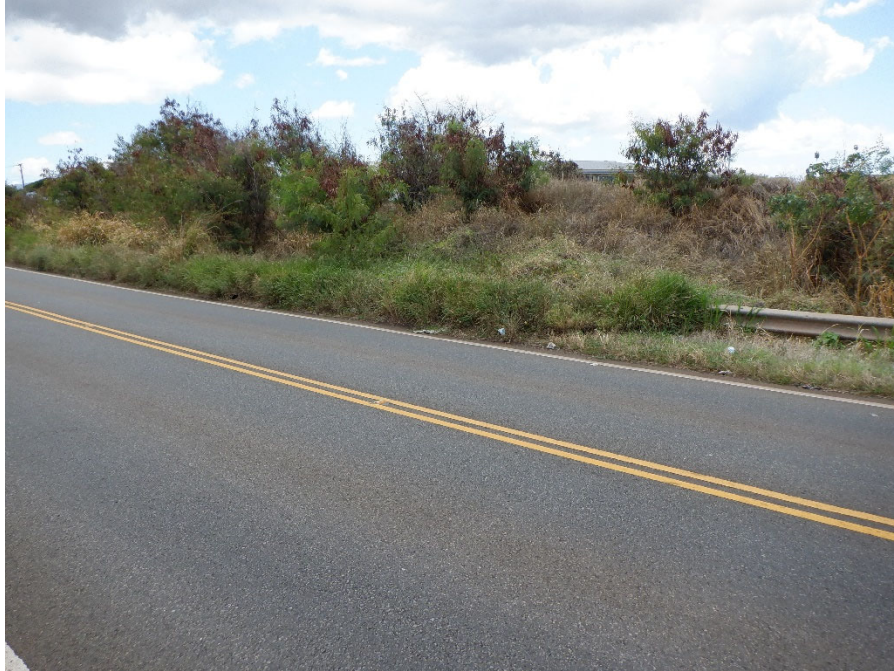
PHOTO 9 DOWNSTREAM EAST APPROACH GUARDRAIL COVERED BY HEAVY VEGETATION
