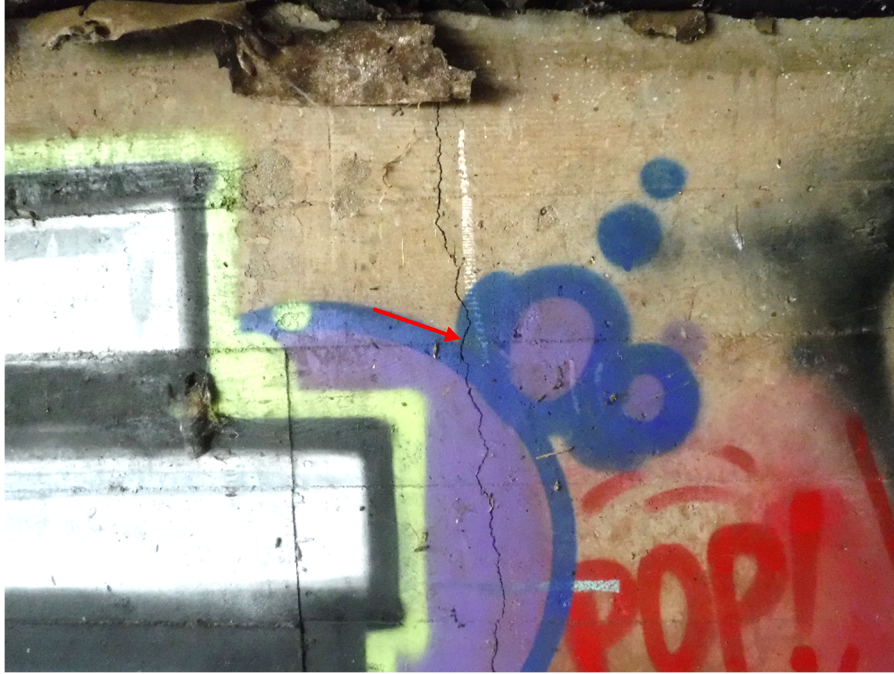
PHOTO 21 WIDE CRACK (1FT 1130 CS3) ON ABUTMENT 1, 25' FROM UPSTREAM END
