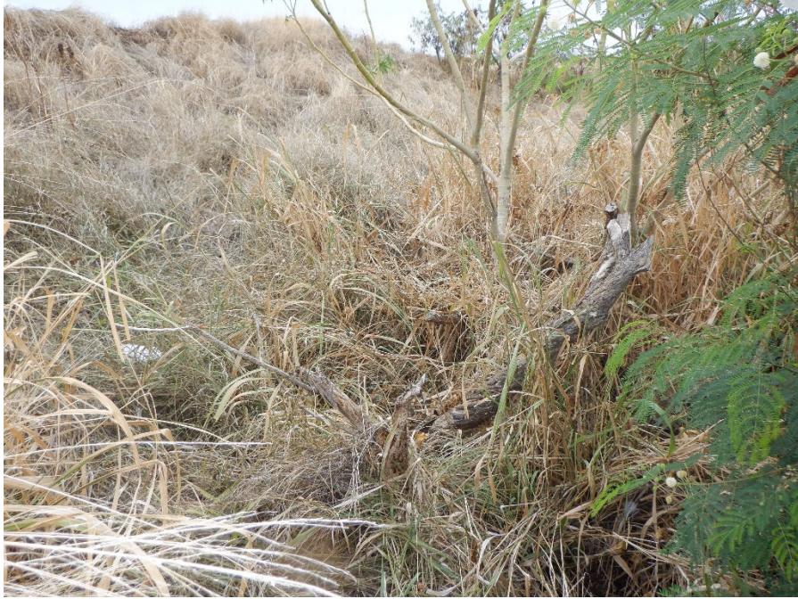
PHOTO 25 DOWNSTREAM CHANNEL WITH HEAVY VEGETATION
