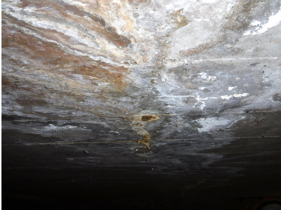
PHOTO 15 LONGITUDINAL CRACK WITH BUILT-UP EFFLORESCENCE (25SF 1120 CS3) ON SLAB SOFFIT, 28' FROM UPSTREAM SIDE
