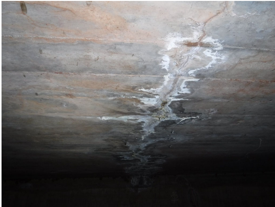
PHOTO 18 LONGITUDINAL CRACK WITH BUILT-UP EFFLORESCENCE (25SF 1120 CS3) ON SLAB SOFFIT, 45' FROM UPSTREAM SIDE
