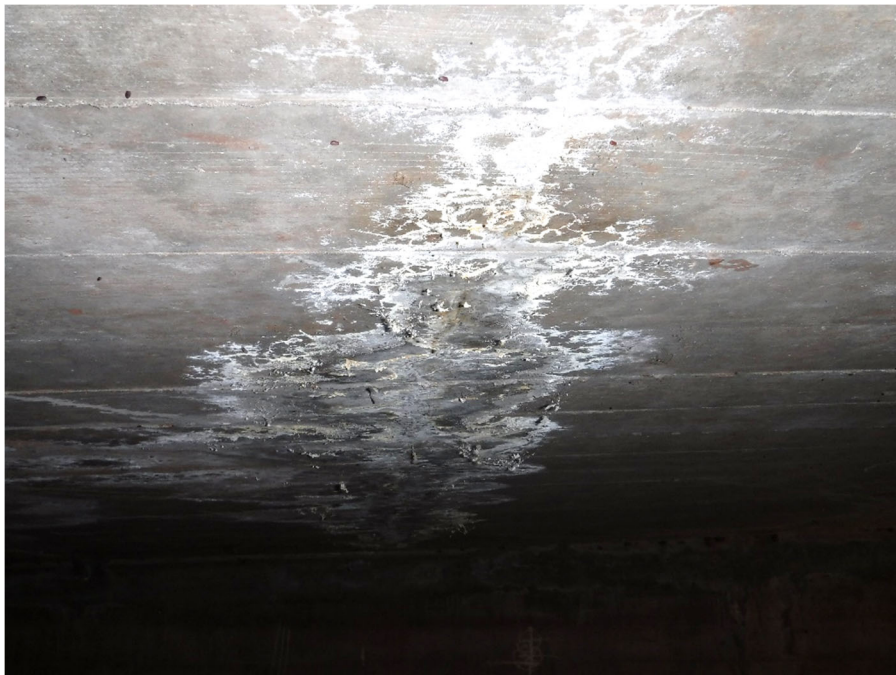
PHOTO 16 LONGITUDINAL CRACK WITH BUILT-UP EFFLORESCENCE (25SF 1120 CS3) ON SLAB SOFFIT, 30' FROM UPSTREAM SIDE
