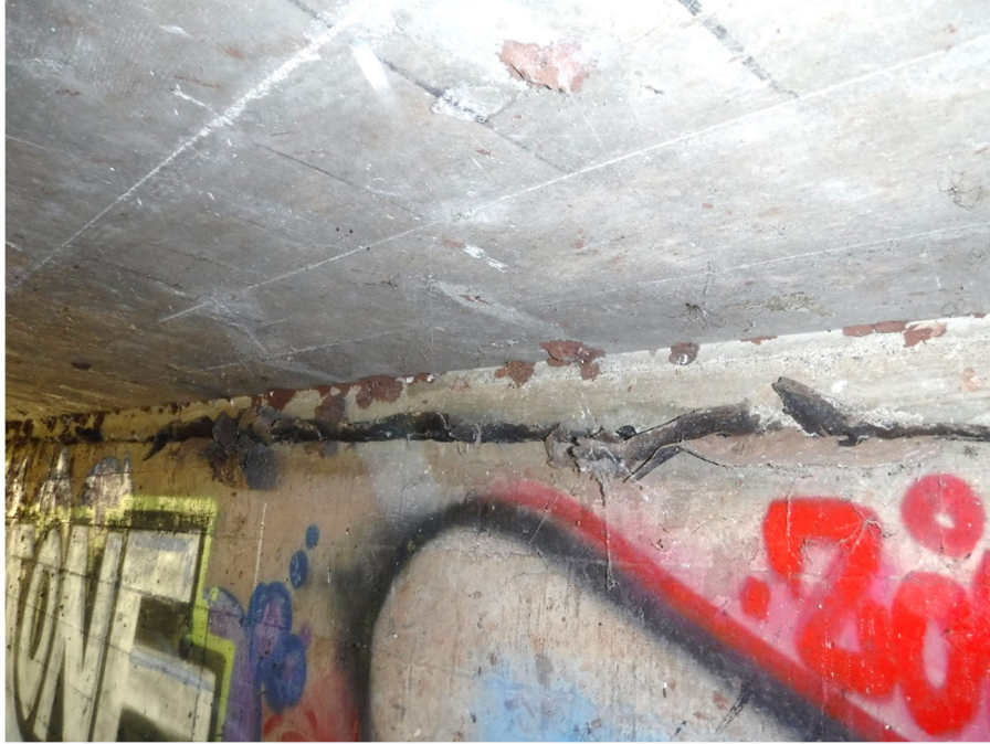
PHOTO 19 PROTRUDING ROOFING PAPER ALONG TOP OF ABUTMENT 1
