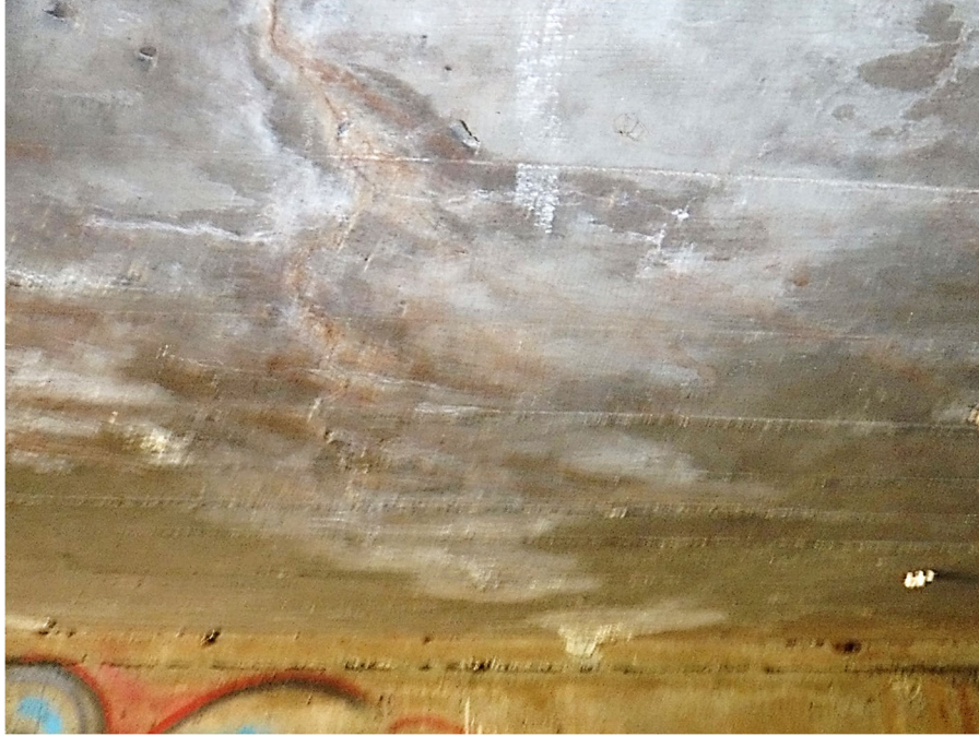
PHOTO 17 LONGITUDINAL CRACK WITH BUILT-UP EFFLORESCENCE (25SF 1120 CS3) ON SLAB SOFFIT, 32' FROM UPSTREAM SIDE
