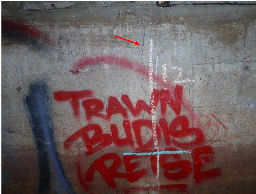
PHOTO 22 WIDE CRACK (1FT 1130 CS3) ON ABUTMENT 1, 45' FROM UPSTREAM END
