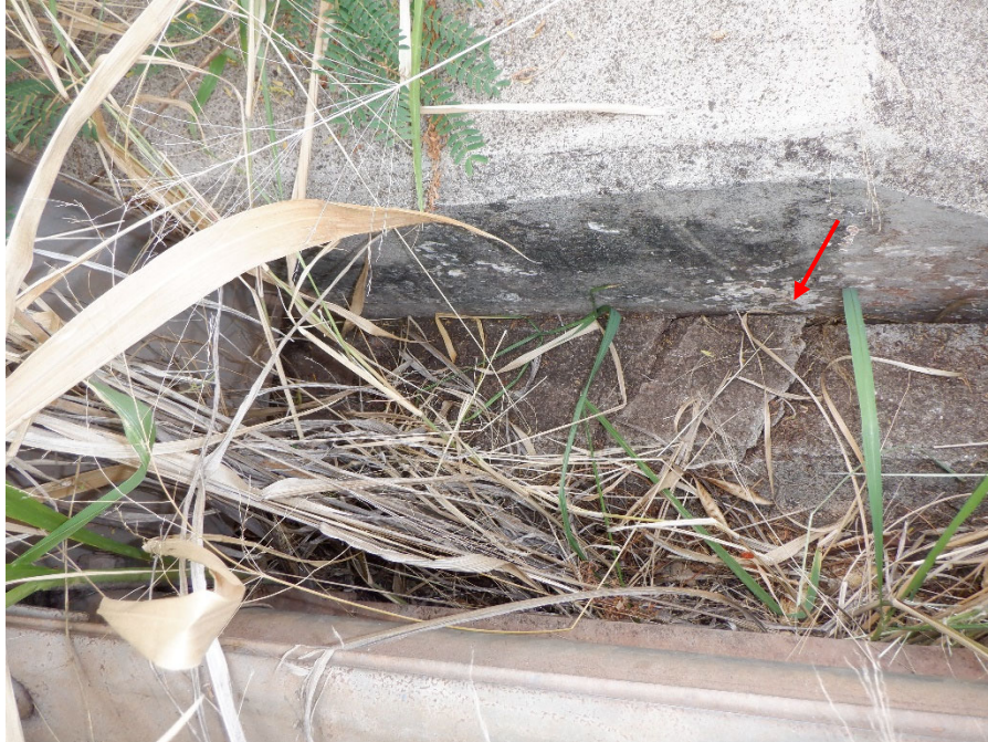
PHOTO 13 2'X1' DELAMINATION ON CURB AT BASE OF DOWNSTREAM CONCRETE BRIDGE RAILING, NEAR WEST END OF BRIDGE
