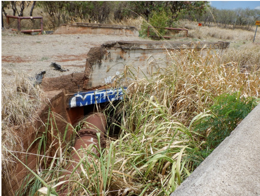
PHOTO 24 UPSTREAM CHANNEL WITH HEAVY VEGETATION AND EXISTING ABANDONED BRIDGE
