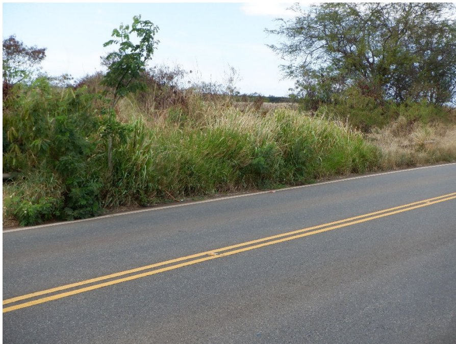
PHOTO 10 DOWNSTREAM WEST APPROACH GUARDRAIL COVERED BY HEAVY VEGETATION
